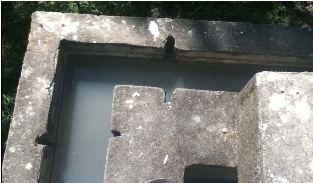
Figure 2.31: Slots for the Control Flow Gates (Walker 2011)
