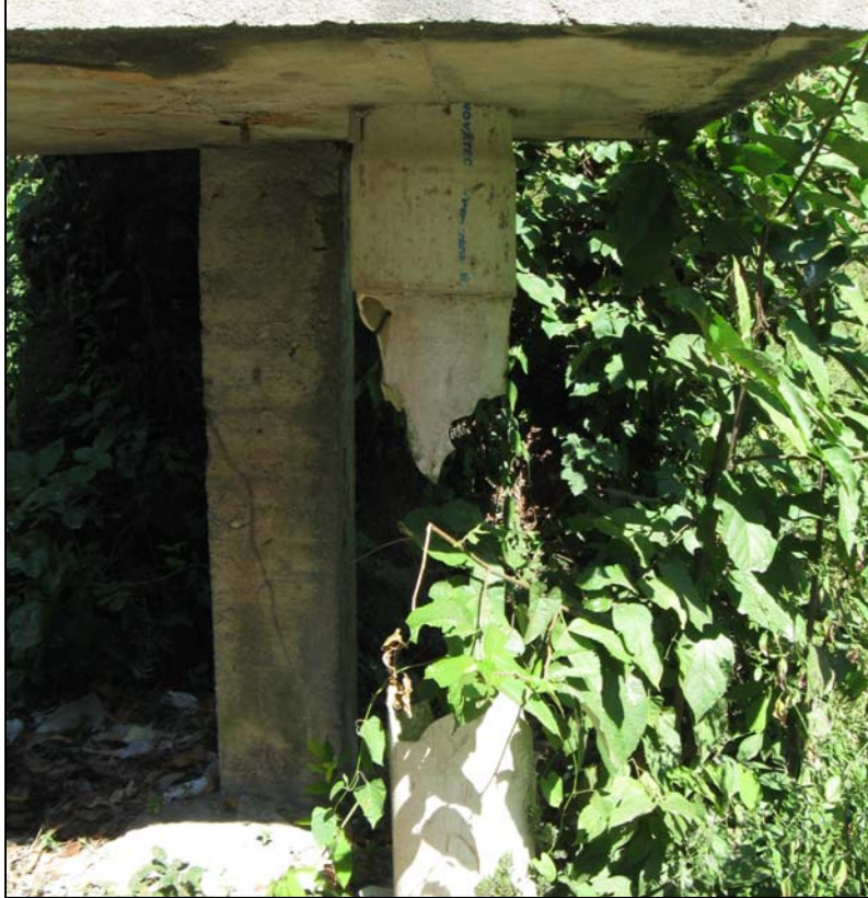
Figure 2.29: Broken Bypass Pipe (Walker 2011)
