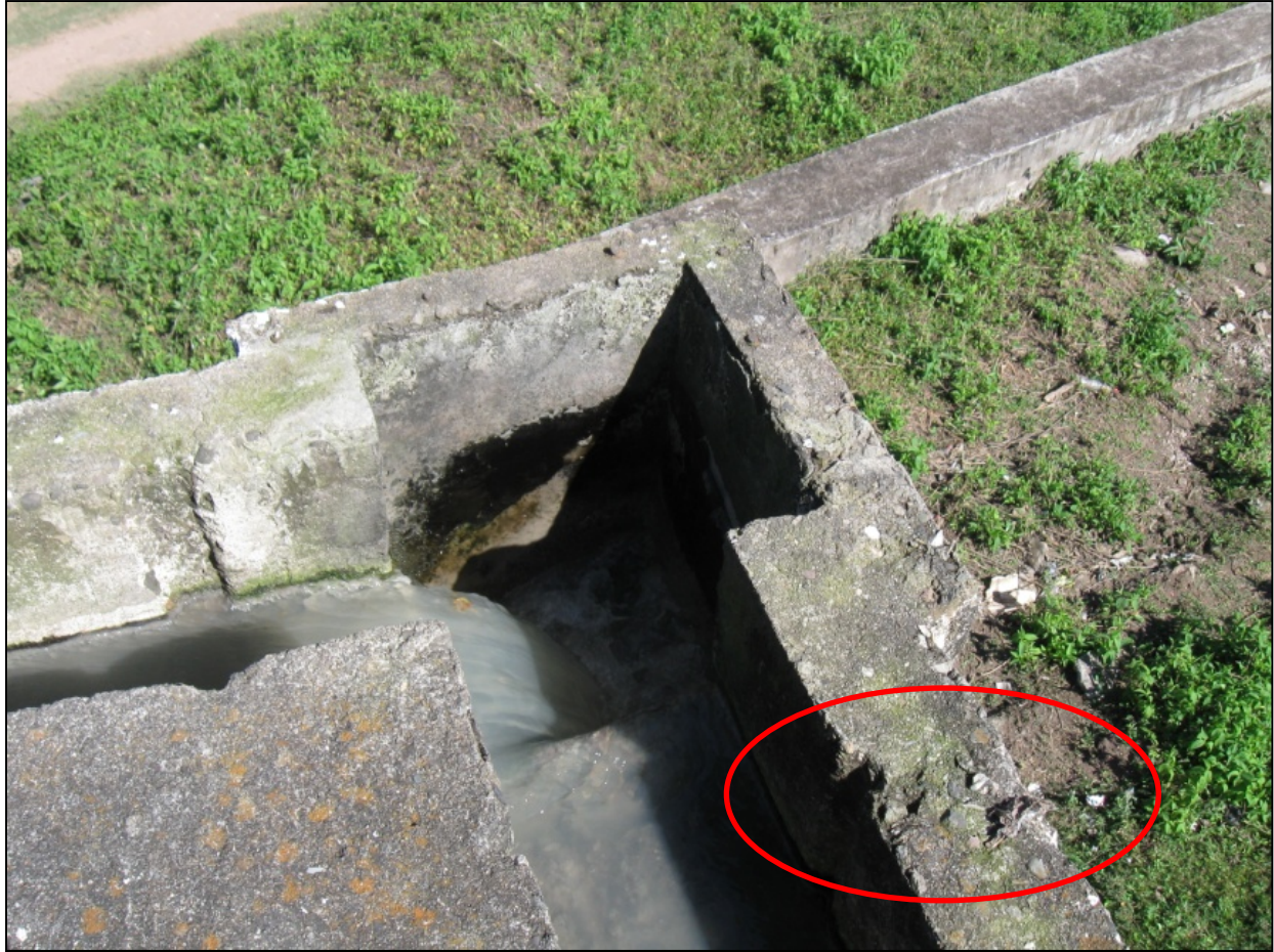
Figure 2.13: Concrete Damage near the Imhoff Tank Outlet (Walker 2011)
