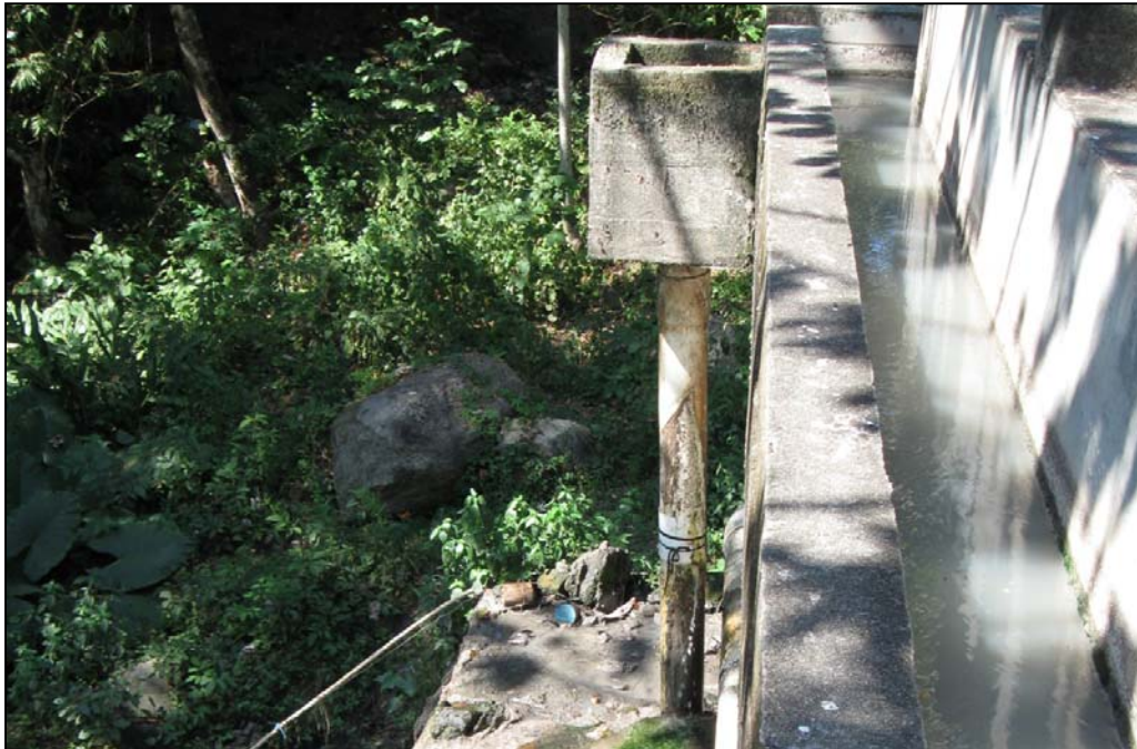
Figure 2.30: Leaky Effluent Pipe (Walker 2011)
