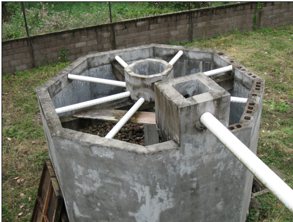
Figure 3.13: Trickling Filter at the Las Casetas Treatment Plant (Puckett, 2011)
