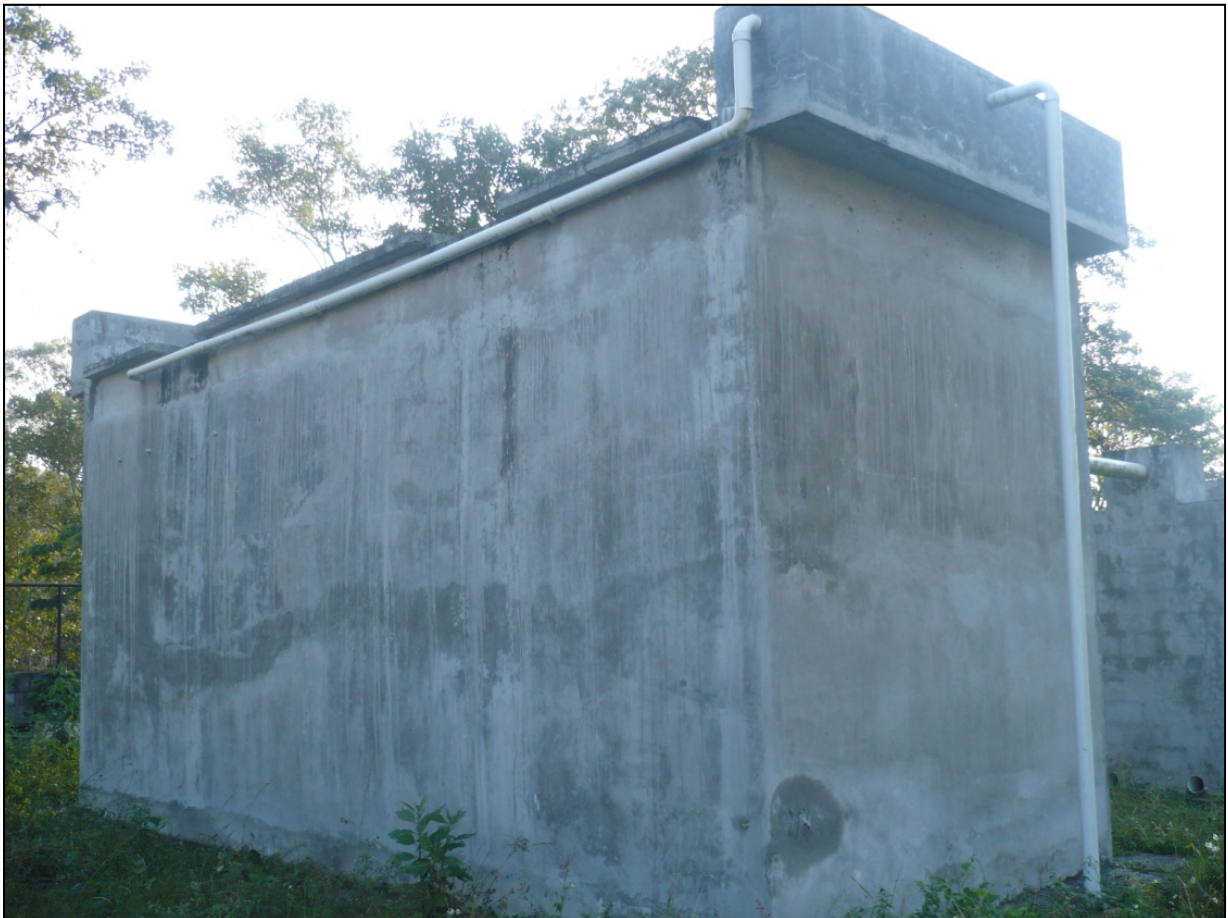
Figure 3.10: UASB Tank at Las Casetas (Walker, 2011)
