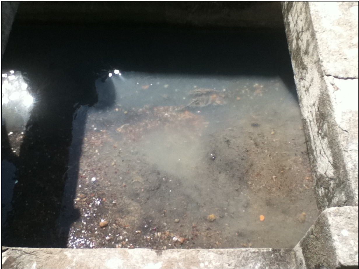
Figure 2.32: Sludge Backup in the First Bay of the Imhoff Tank (Walker 2011)
