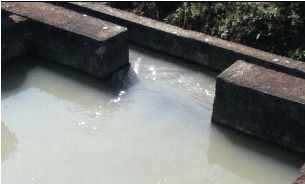
Figure 2.18: Uneven Flow into First Battery of the Imhoff Tank (Walker 2011)
