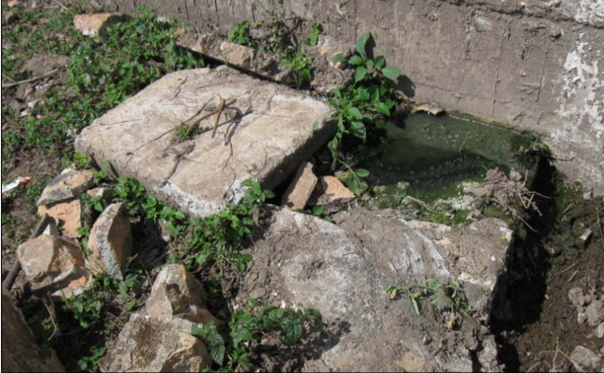
Figure 2.20: Location of Missing Sludge Valve (Walker 2011)
