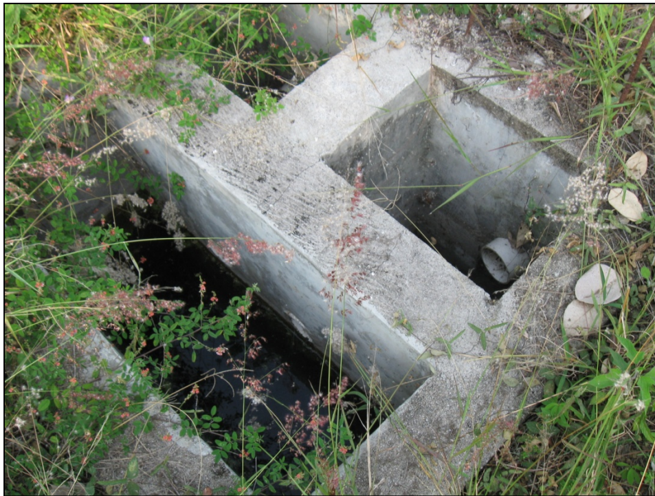
Figure 3.22: Distribution Box Between Trickling Filter and Secondary Clarifier (Puckett, 2011)
