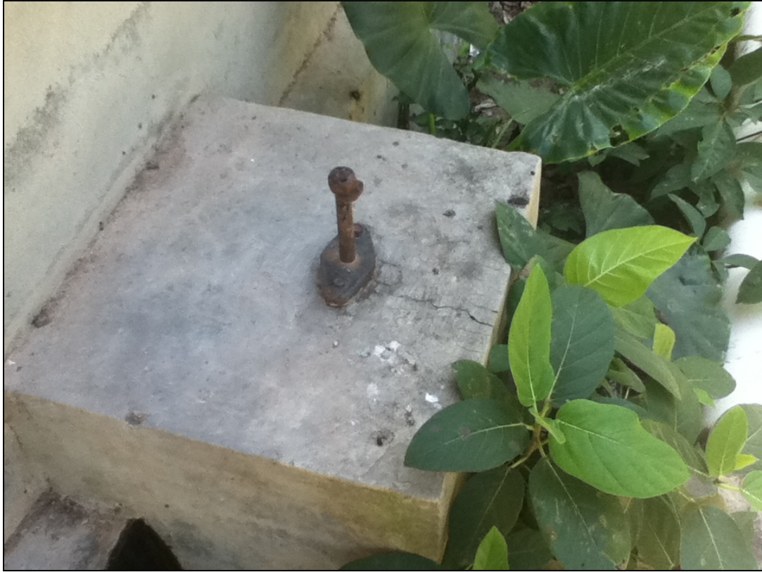
Figure 2.33: Missing Sludge Valves (Walker 2011)
