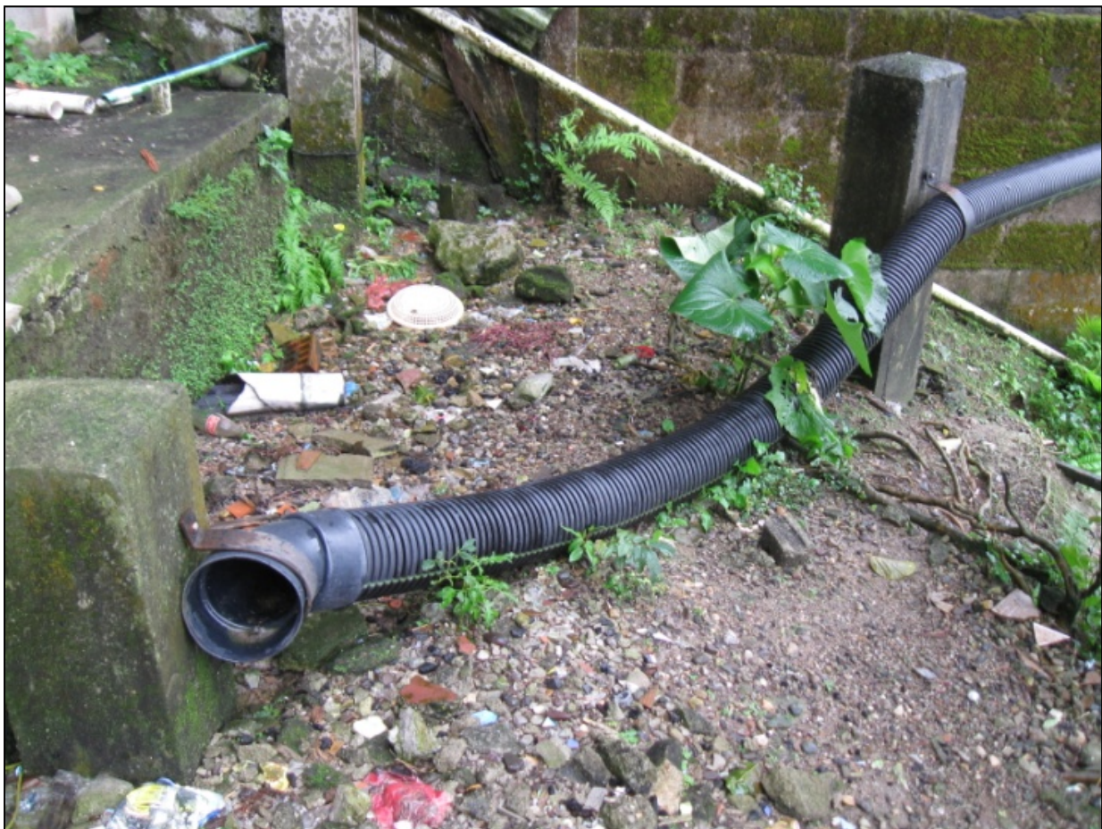
Figure 3.2: Current Condition of Piping System (Walker 2011)
