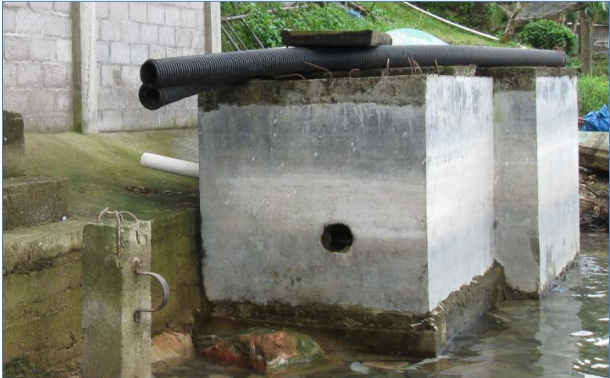
Figure 3.5: Distribution Tank (Walker 2011)
