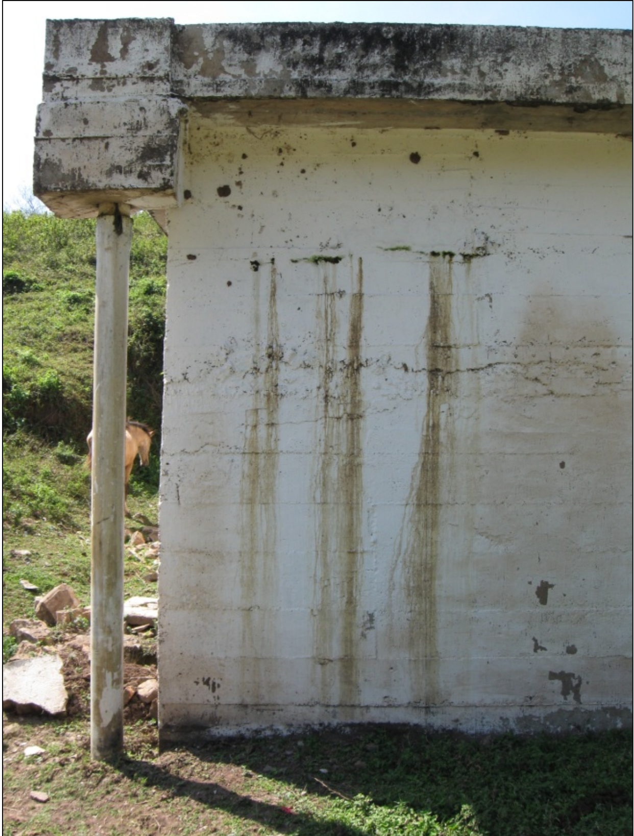
Figure 2.12: Effluent PVP Pipe (Walker 2011)
