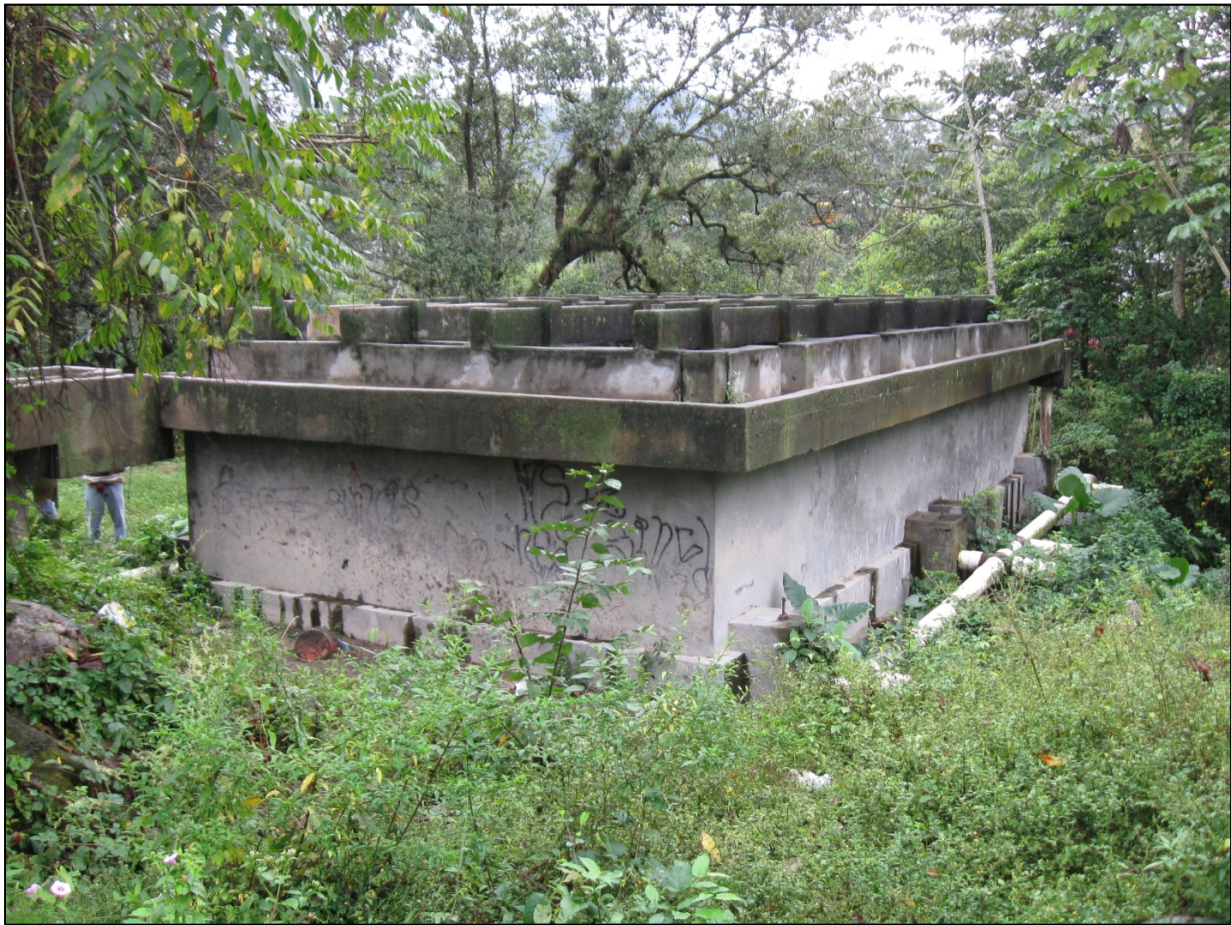
Figure 2.26: Santa Barbara Imhoff Tank (Puckett 2011)
