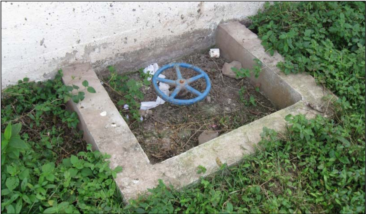
Figure 2.21: Sludge Valve (Walker 2011)
