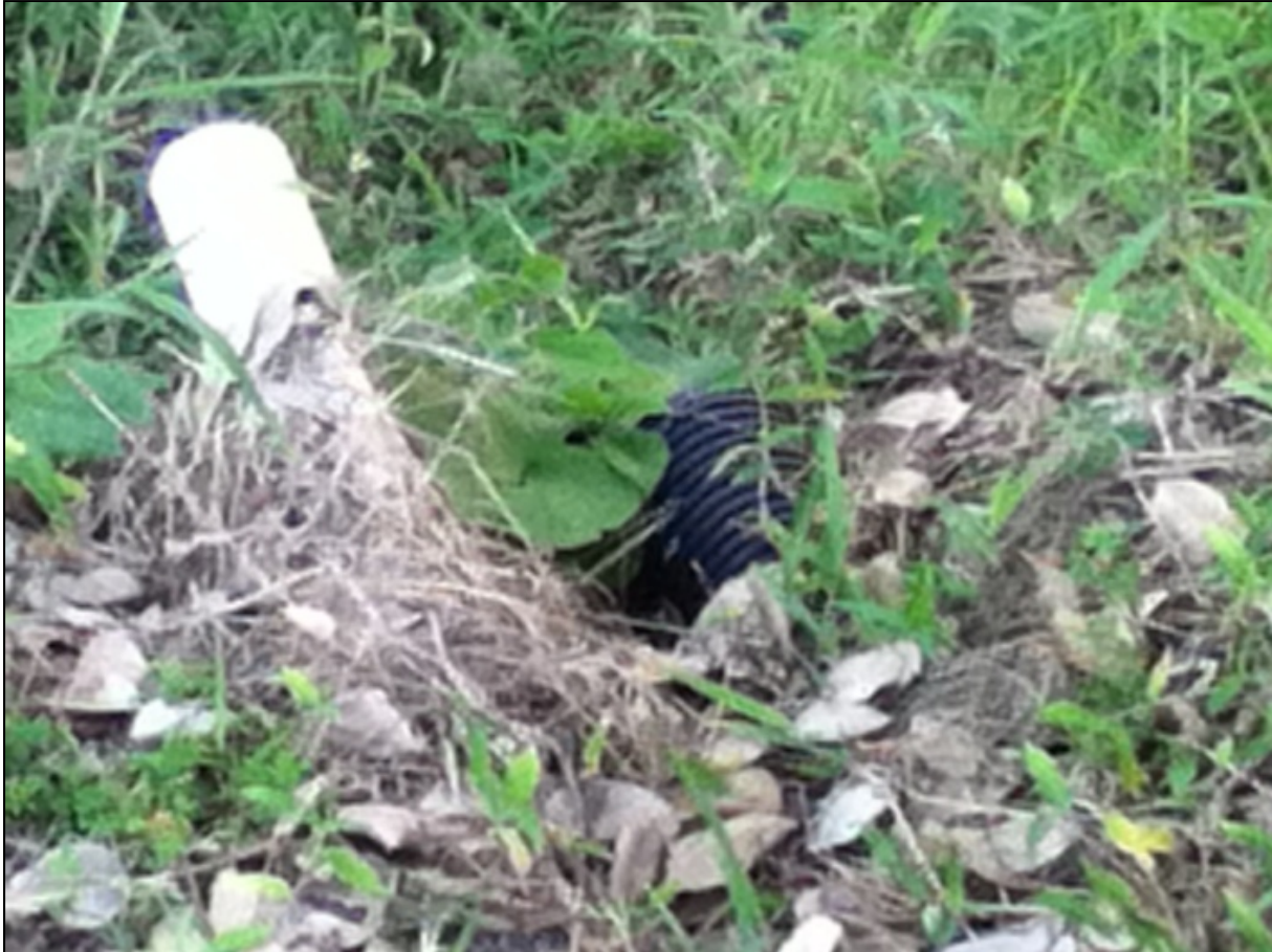
Figure 3.1: Influent and Effluent Pipes just Outside the Treatment Plant (Walker 2011)
