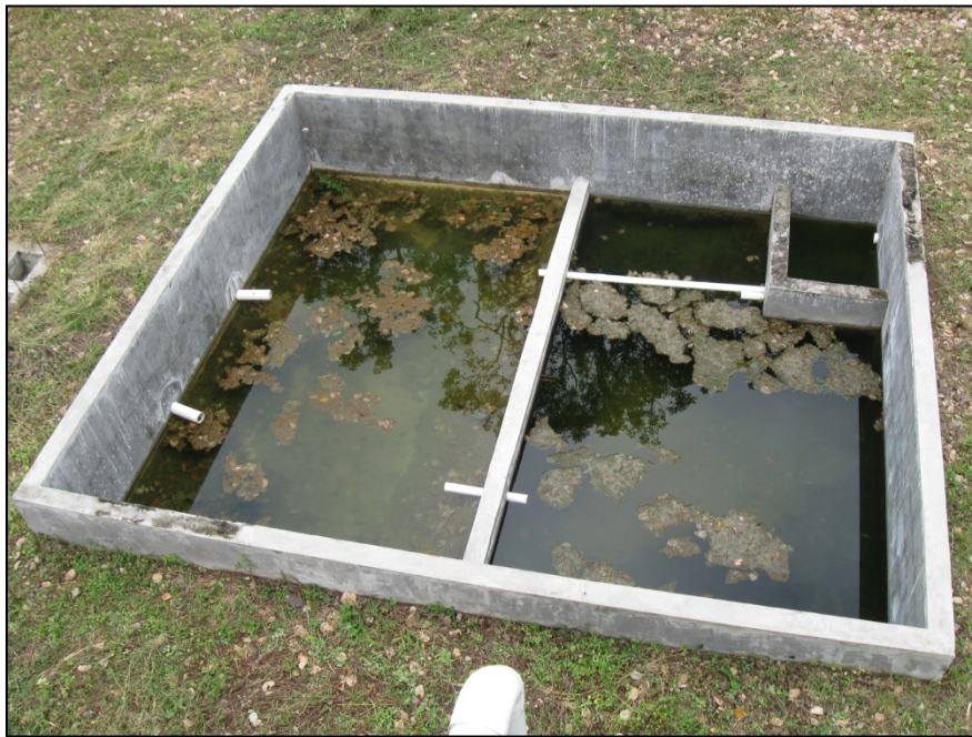
Figure 3.19: Secondary Clarifier at Las Casetas Treatment Plant (Puckett, 2011)
